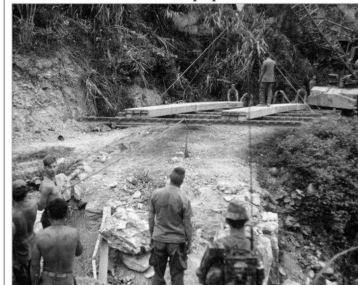
Marine engineers repair a bridge along Route 9 near Khe Sanh. In April 1968, Operation Pegasus successfully relieved the beleaguered combat base and reopened Route 9 for traffic. (Courtesy of the USMC Vietnam Tankers Association)
